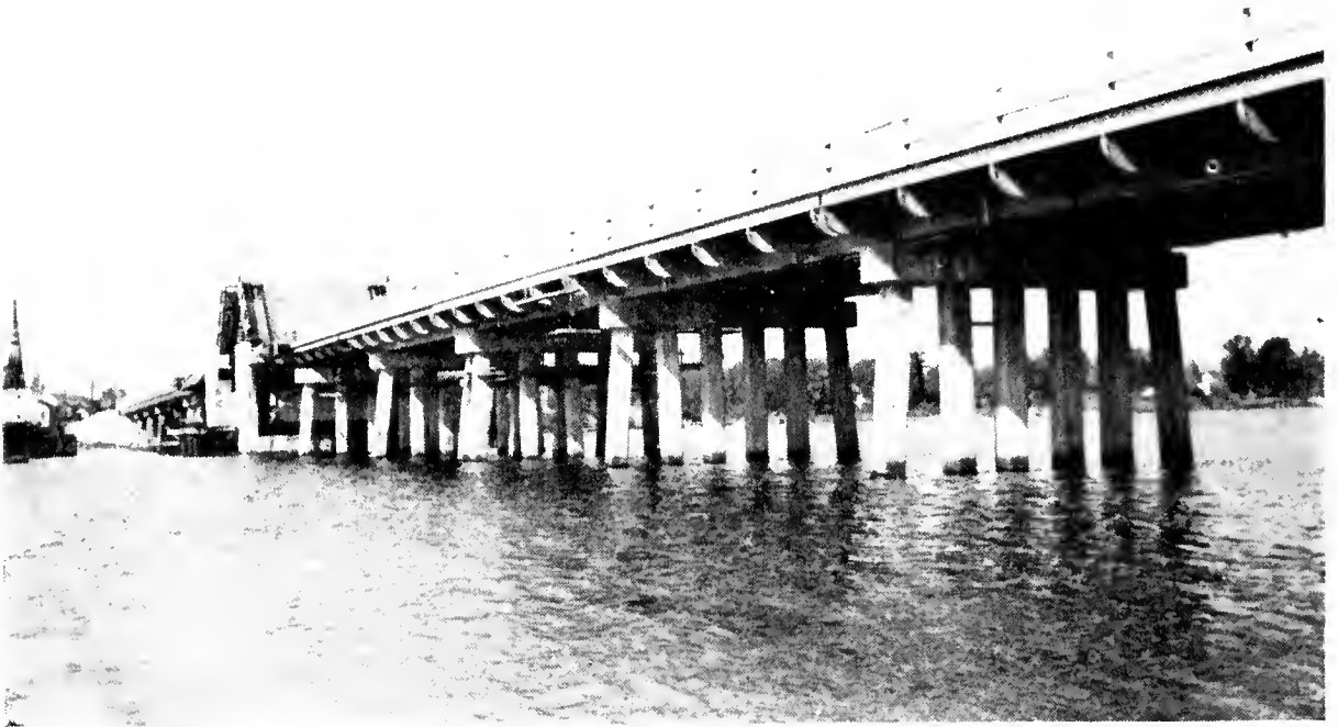
BRIDGE OVER STONY CREEK ON FORT SMALLWOOD ROAD, NEAR RIVERA BEACH, ANNE ARUNDEL COUNTY. UNDER CONSTRUCTION JUNE 30, 1948
